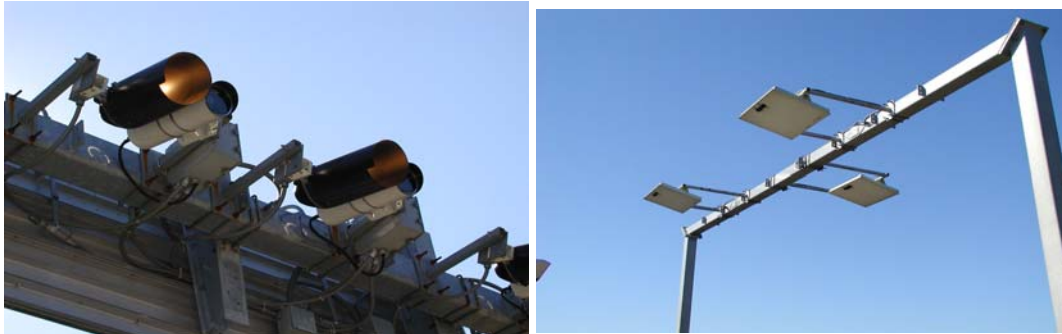
Figure 3-54: Example of Overhead RF Antennae Used with AVI (right) and Cameras Mounted at a Tolling Installation (left)
